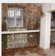
On damp masonry
