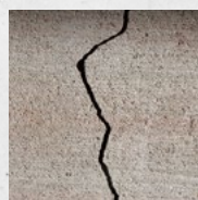
For dry cracks
